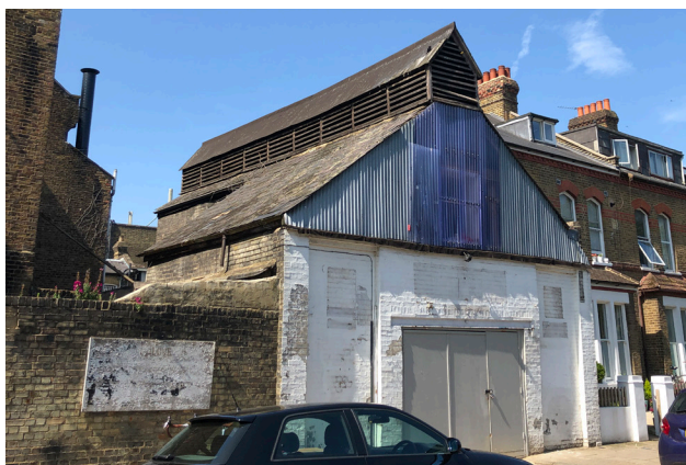
Fig 5.5 108 Finsbury Park Road
